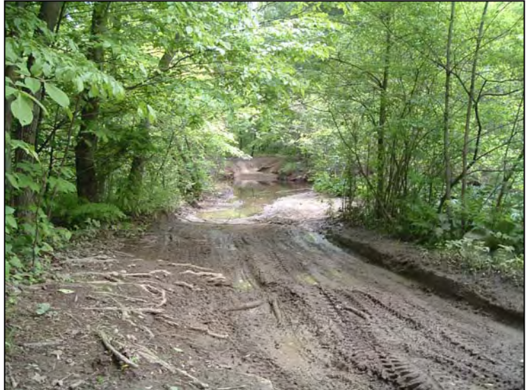
ATV damage in Bear hole Reservoir - June, 2005
