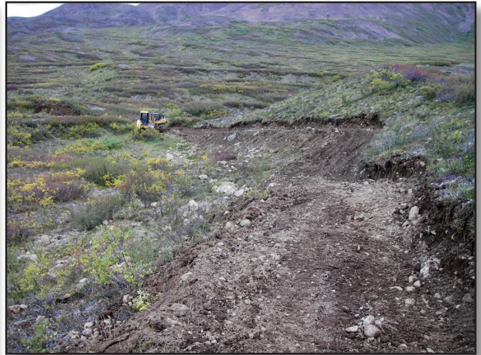
Trail specifications included contour curvilinear alignment, controlled average grade (not to exceed 10 percent), and integrated water control.
