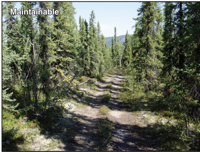
Figure 3-3—An example of a maintainable trail section in the Fortymile River area, AK. This section has a contour alignment and an average trail grade less than 10 percent, but it lacks adequate water control. Rolling grade dips could be integrated into the alignment for increased sustainability.
