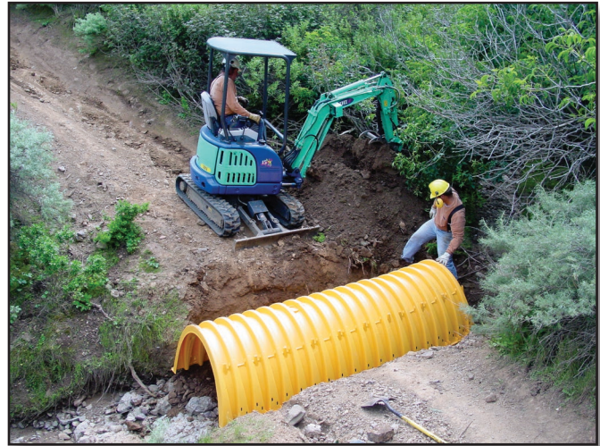
Figure 14–2—A miniexcavator is a versatile piece of equipment for trail construction and maintenance and plays a valuable role in supporting trail dozer operations.
