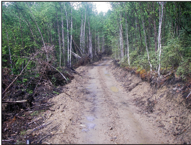
One of the areas where the Sweco 480 was used to directly clear timber from the alignment. Note the trees pushed into the forest.
