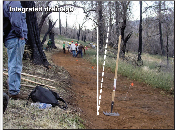
Figure 2-3—Note the angle of the trail tool handle. It shows that the trail tread has outslope, one type of integrated drainage (the third sustainable trail design guideline). Outslope encourages water to flow across the trail. Unfortunately, functional outslope is usually lost on off-highway vehicle trails when wheel ruts form. Grade reversals and rolling dips overcome this problem.
