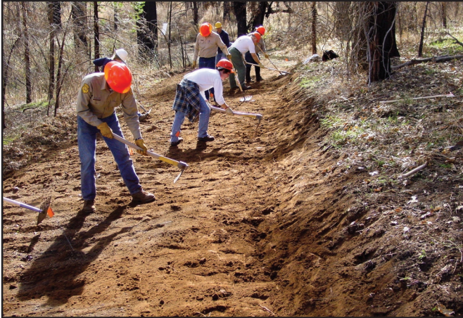
Figure 12-1—A trail crew uses handtools to shape the final tread surface to meet the design specifications.
