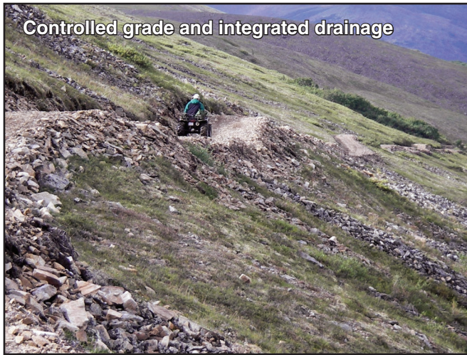
Figure 2-2—This off-highway vehicle trail in the Bureau of Land Management White Mountains National Recreation Area illustrates controlled grade and integrated drainage, the second and third sustainable trail design guidelines. Note how the trail slowly descends the sidehill. In this case, the grade never exceeds 10 percent and grade reversals (short, abrupt changes in grade) serve as integrated water control features. The all-terrain vehicle rider visible in the photo is traversing the bottom of one of the grade reversals.
