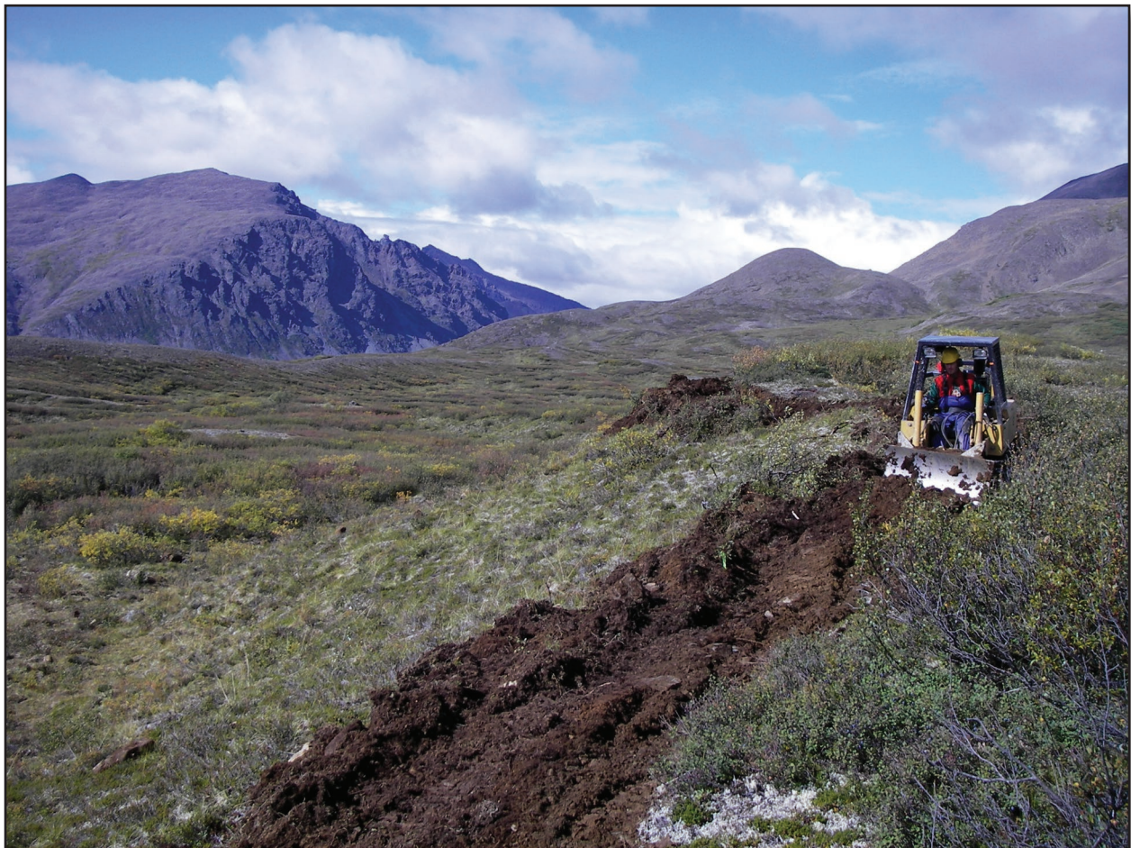
A Sweco 480 trail dozer roughs out the trail bench on the Glacier Lake Trail above Rock Creek. The Sweco 480 is specially designed for trail work. It has a track width of 4 feet and a six-way blade that is 5 feet wide. Jon Underwood of Happy Trails, Inc., Fairbanks, AK, was the owner/operator for the project excavation.
