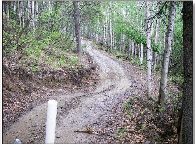
One of the many grade reversals integrated into the trail alignment to make sure that water flows on average for no more than 100 feet along the tread surface.
