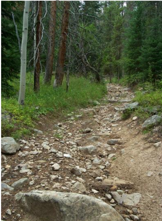
Erosion damage to Single Tracks
